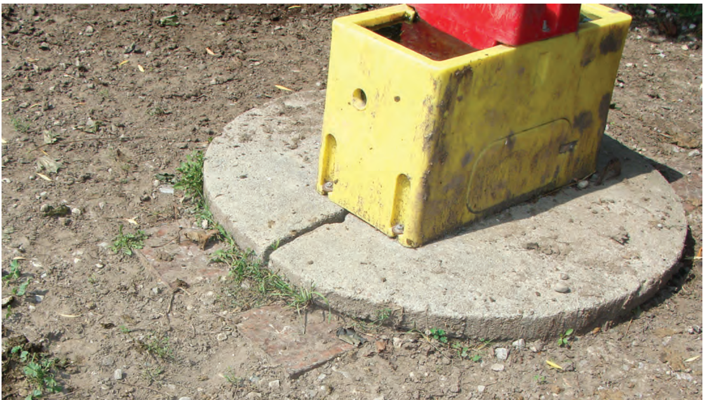
This picture shows the gap in the concrete well cap and its location in relation to the ground and potential sources of contamination.
