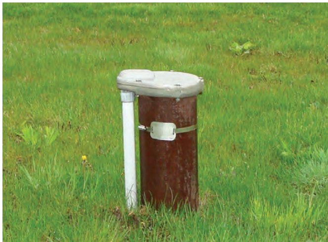
Properly constructed drilled well shown with a vented and vermin proof well cap, electrical conduit for submerged pump (to left of well casing), identification tag (linked to Water Well Record), casing extends at least 40 cm above the ground, and ground that is mounded away from well casing.
