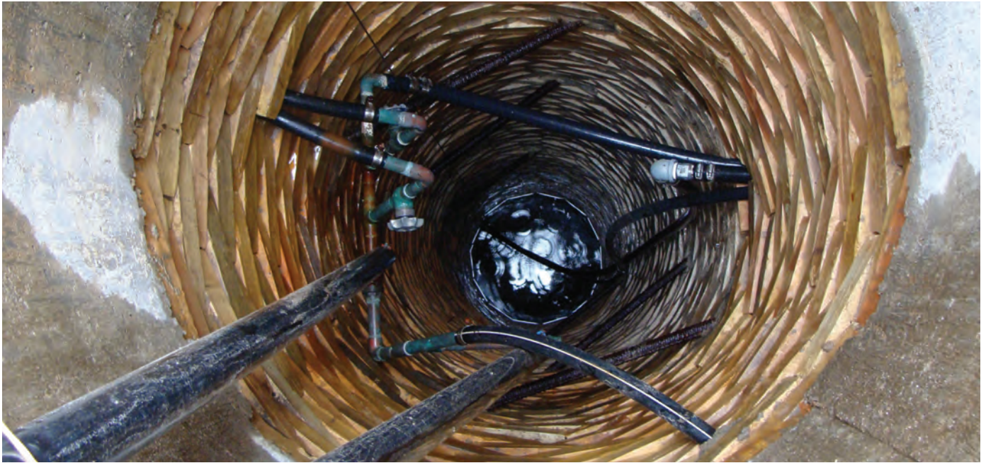
A dug well that is over 100 years old. Moisture seen on the concrete and tile casings indicates that surface water is getting into the well. Ensure that the well is constructed and maintained properly to reduce potential contamination from entering the well.
