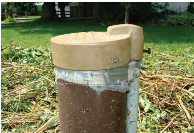
An inadequate well cap may allow pests and other types of contamination to enter into the well, and may not allow for proper ventilation.
